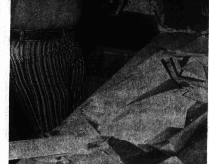
SIGNS OF UNWELCOME VISITORS — Mack Gamble, general manager of Town & Country Shopping Center, U.S. 87 South, surveys the damage caused by thieves who broke into the center over the weekend, taking approximately $80 in cash. Entry was gained through a hole knocked in the south wall of the shopping center.
