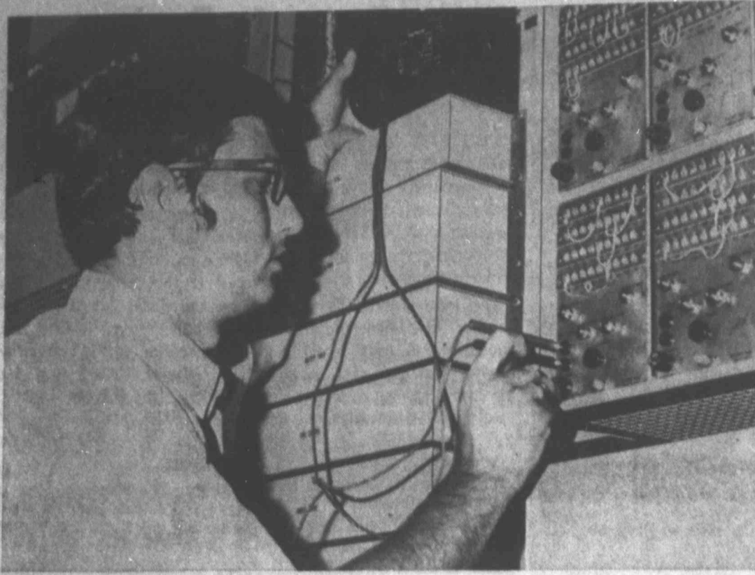
NEW PHONE SERVICE — Shown checking some of the central office equipment at the General Telephone Company's new exchange building in Forsan is Donald R. Baker, equipment installer. The new exchange and DDD service is scheduled to go into service Sept. 19.
