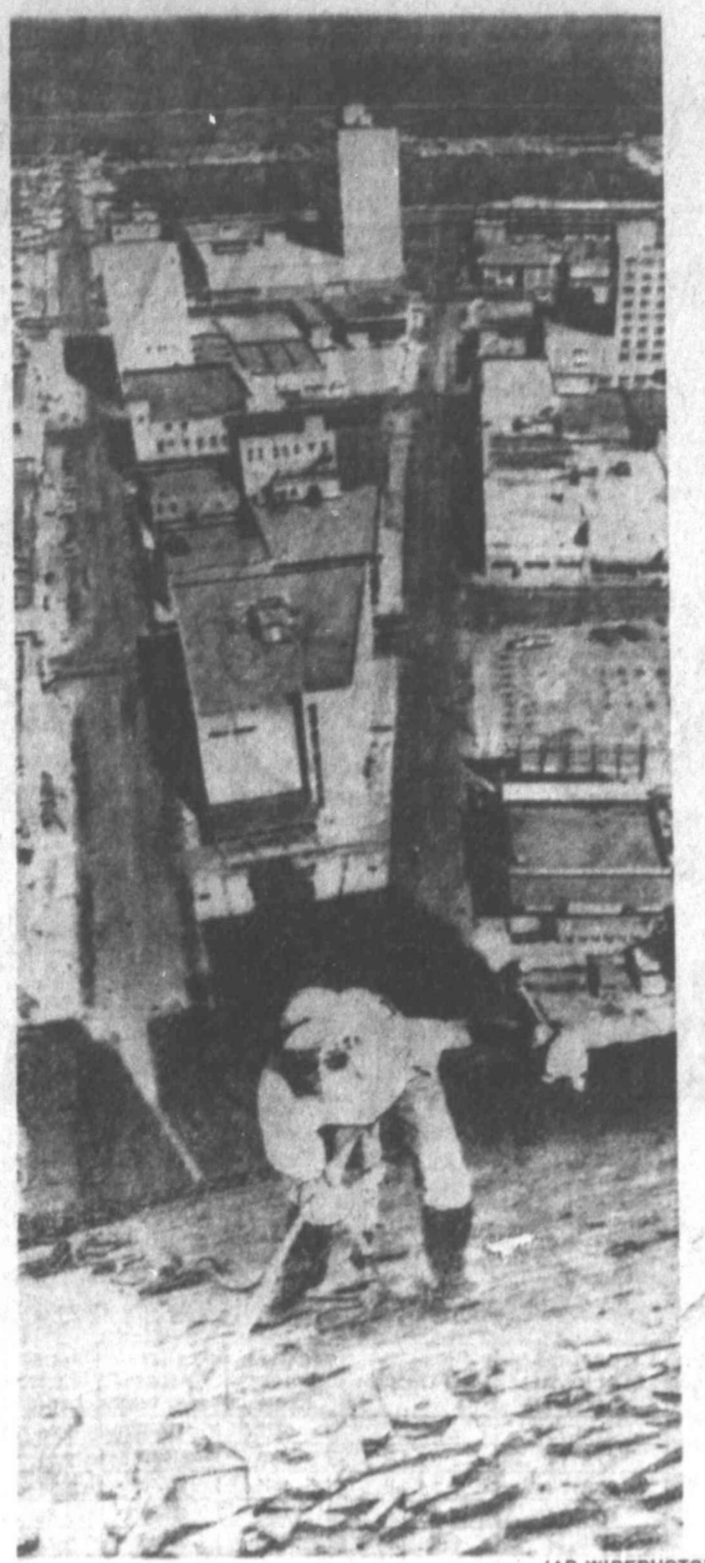
ABOVE IT ALL — John Rogers of Corpus Christi spent most of his day Tuesday laboring atop the Driscoll hotel several hundred feet above earthbound passersby. Rogers was knocking roofing material off the roof of the closed hotel which will be converted into an office building. Photographer George Congora tied himself with a rope so he could get this angle.
