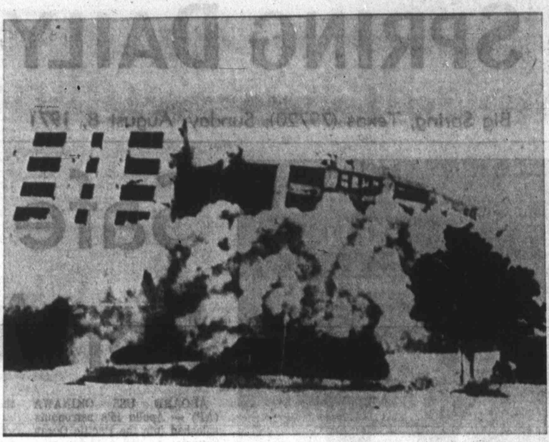
LANDMARK OBLITERATED — The once majestic Edgewater Gulf Hotel at Biloxi, Miss., a favorite watering hole for the wealthy in the 1930s, relinquished its last structural hold on property destined for a shopping center here as dynamite reduced its last standing wing to rubble and dust. The old hotel, which had hosted guests such as President Harry Truman and New York Mayor Jimmy Walker, was subjected to two earlier blasts, each claiming a portion of the eight-story structure.
