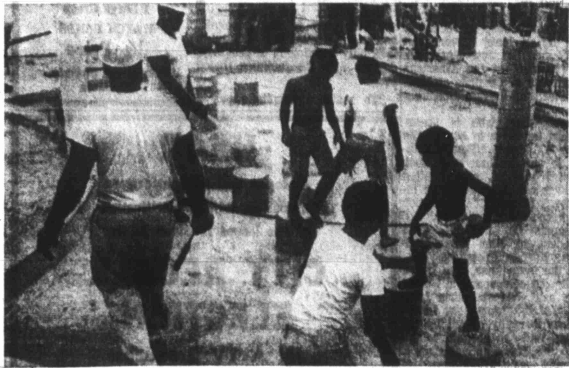
WORKMEN AND KIDS IN SPLASHPool — Four youngsters hop from one stepping stone to another trying out the new splash pool even while laborers are still working on the mini park being built in the center of Miami's ghetto area. The tiny park is an experiment in transforming a city lot into a park with most of the labor being donated.
