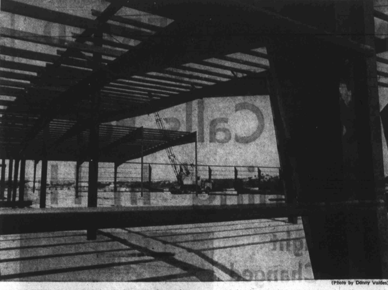
MOBILE HOME PLANT TAKING SHAPE — Workmen plan to have the remainder of the iron framework for Eagle Mobile Homes up by the end of this week. Leo Koestler, plant manager, said the plant should be finished in about three weeks, and he hopes the plant will be turning out its first mobile home by the first of August.
