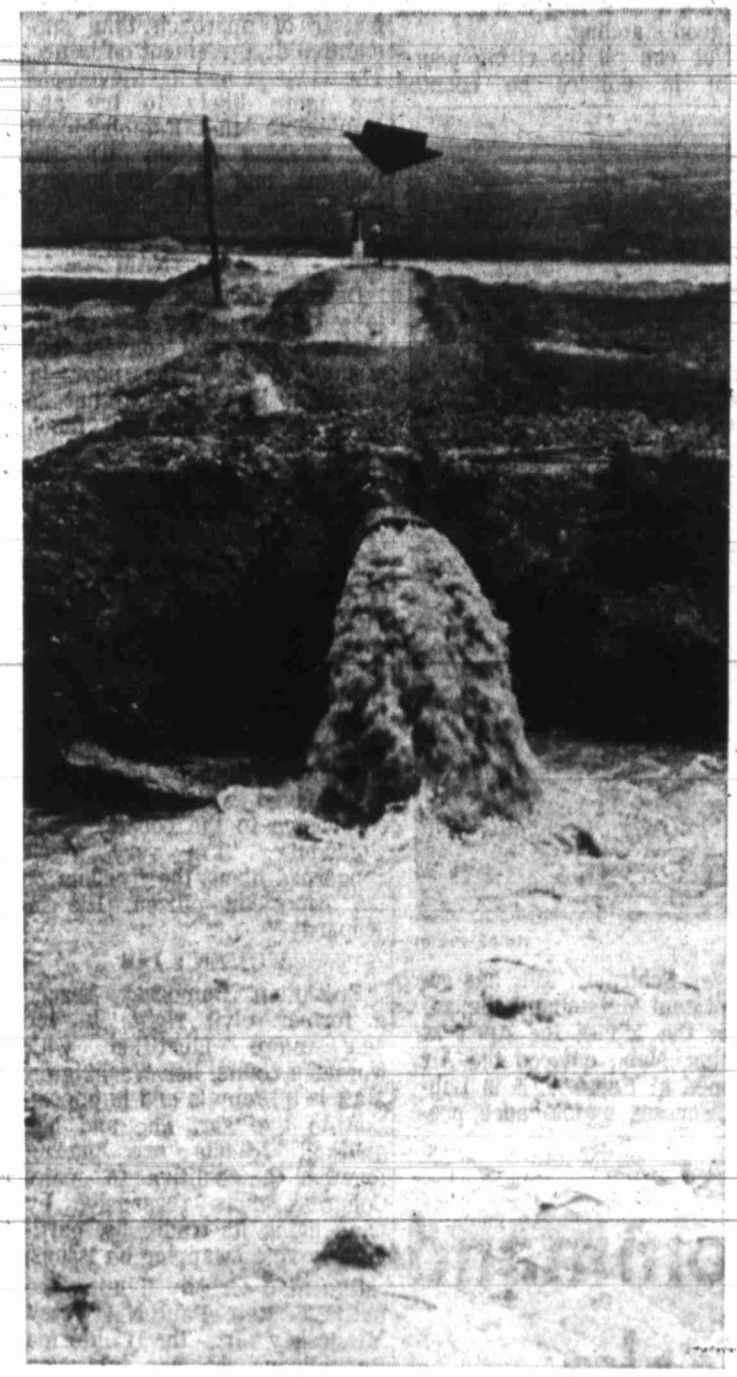
PUSHING WATER UP THE STEPS Arrow indicates pump in river channel
