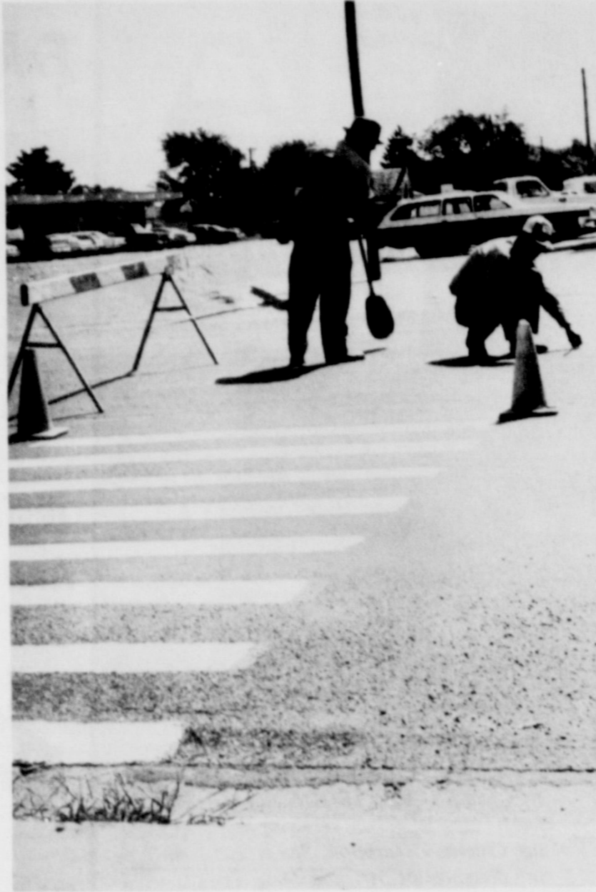
PAINTING WALKS... City of Friona employees are shown painting the crosswalks on Main Street, in preparation for the upcoming school term, which gets underway August 27.
