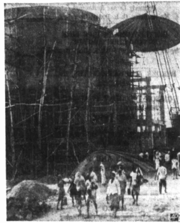
OLD AND NEW —Bamboo is still used by workers as scaffolding for this pulp plant storage tank, made in part of fiberglass-reinforced plastic, at site in India.
