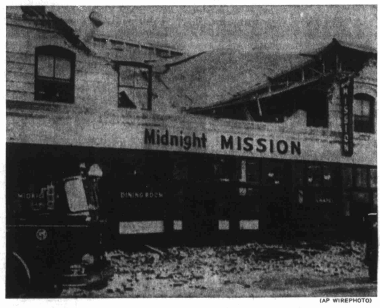
SCENE OF CALIFORNIA EARTHQUAKE DEATH — Rubble from a partially collapsed building at the Midnight Mission near the skid row section of downtown Los Angeles marks the area where at least one man was killed today in a strong earthquake.
