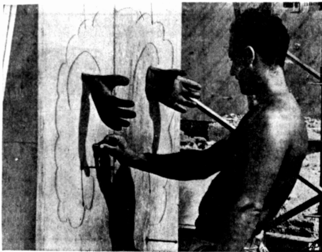
CONCRETE HANDIWORK — No one is buried in this concrete wall construction project at Wilmington, Del. One of the workmen stuck his gloves on metal tie rods which project through the concrete and worker Joe DeFilippa went along with the gag.
