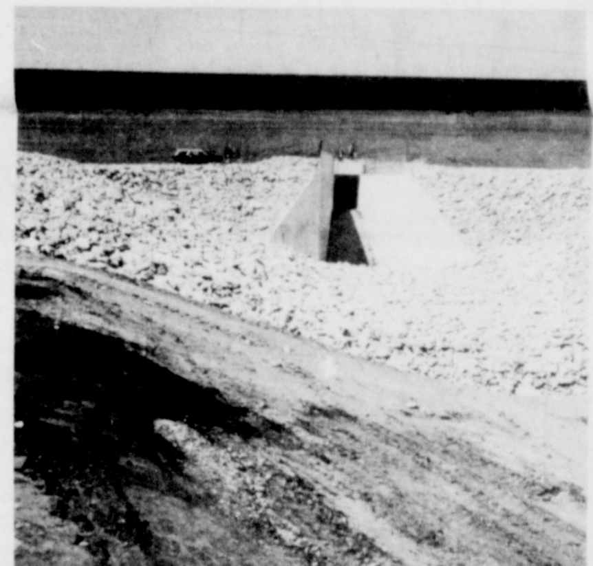
SPILLWAY.... An idea of the size of the spillway on the new dam on Running Water Draw is seen in this shot. The spillway opening measures eight feet by eight feet.
