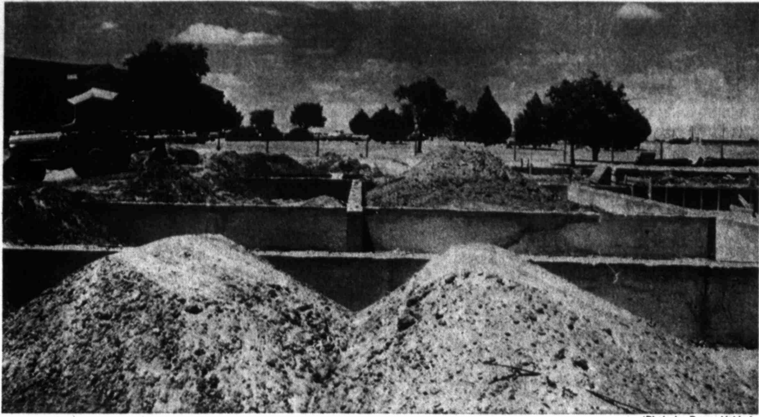
FOUNDATIONS FOR CHAPEL LAID — Construction on All-Faith Chapel at Big Spring State Hospital is almost 20 per cent complete with final pouring of foundations set for this week. The $129,131 facility could be completed ahead of the
