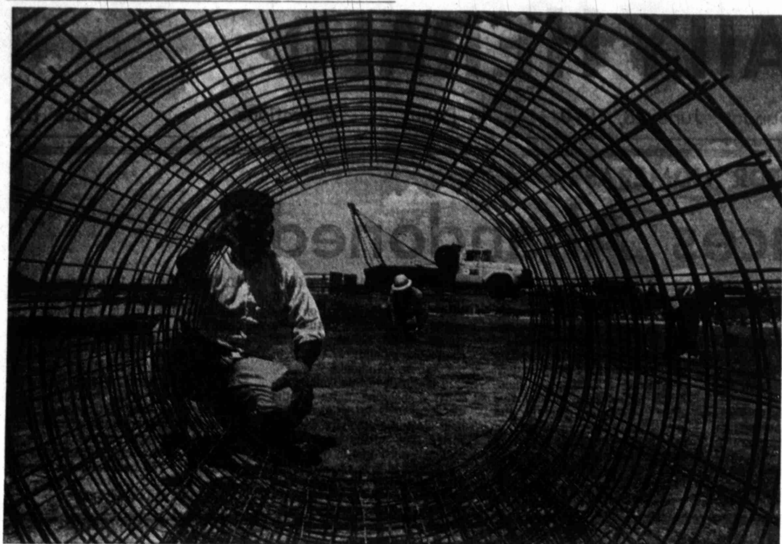
BULLSEYE FOR NEW FACILITY — Reinforcing steel forms a bullseye for the new Intech facility which is beginning to take shape at the west edge of Big Spring. Last week five local sub-contractors were let for plumbing, mechanical, site
