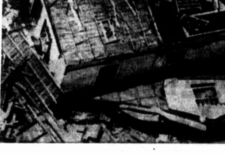
ROOFLESS HOUSE — A powerful tornado which struck Monday night lifted the roof off this house in the residential district of Lubbock. The twister killed 21 persons and injured hundreds. Damage is estimated to go into millions of dollars.
