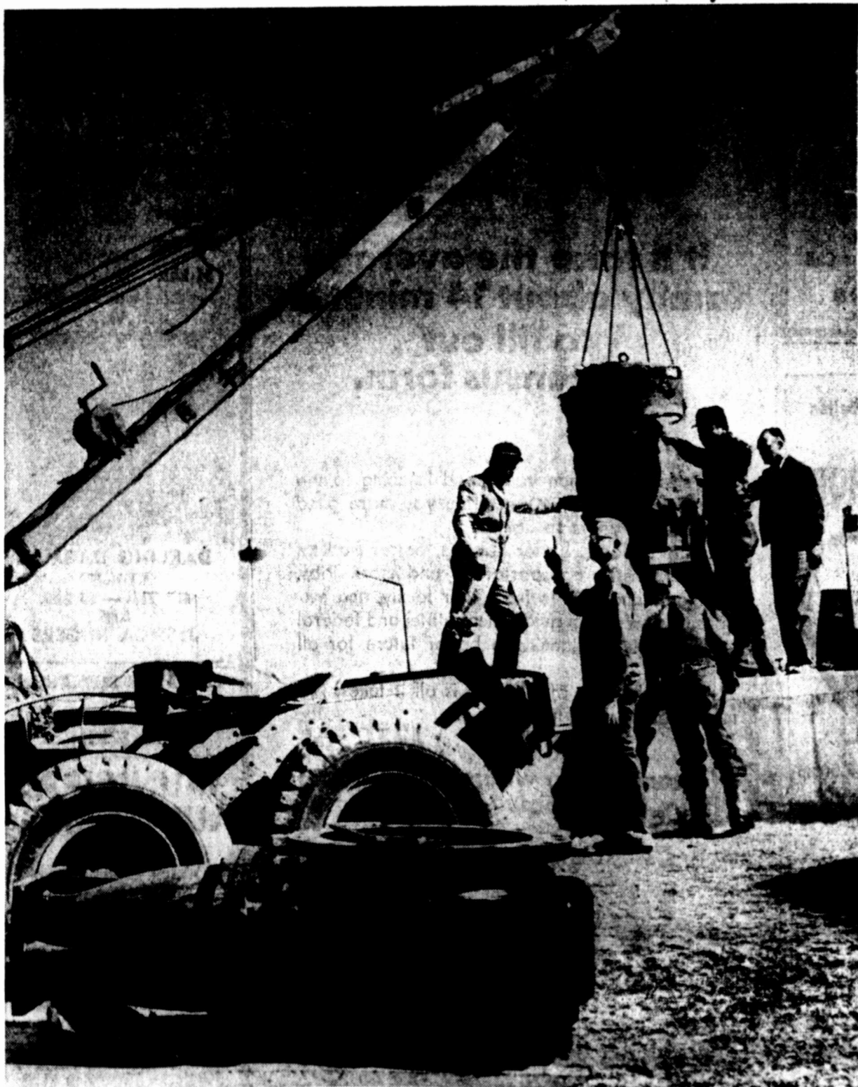
CHECKING CONSTRUCTION —Every time any work was done around the water plant, Roy Hester was on hand to see that it was done right. Here, concrete was being poured at the new clearwell at the water treatment plant, a project of the City's Master Plan capital improvements.
