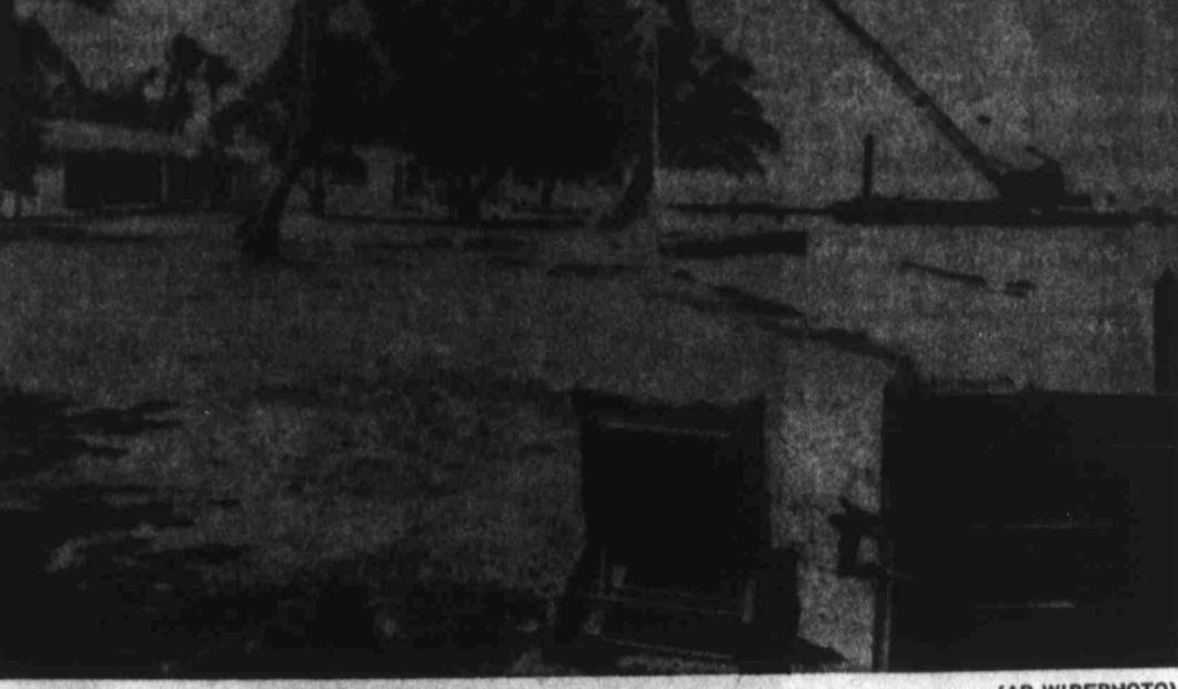
PRESIDENTIAL PAD IN THE MAKING — Crane and piler work on landing pad for helicopters just offshore in Biscayne Bay last spring at President Nixon's compound at Key Biscayne, Fla. It was reported Friday that U.S. Army Engineers spent $342,358 to build the 150-foot square pad.
