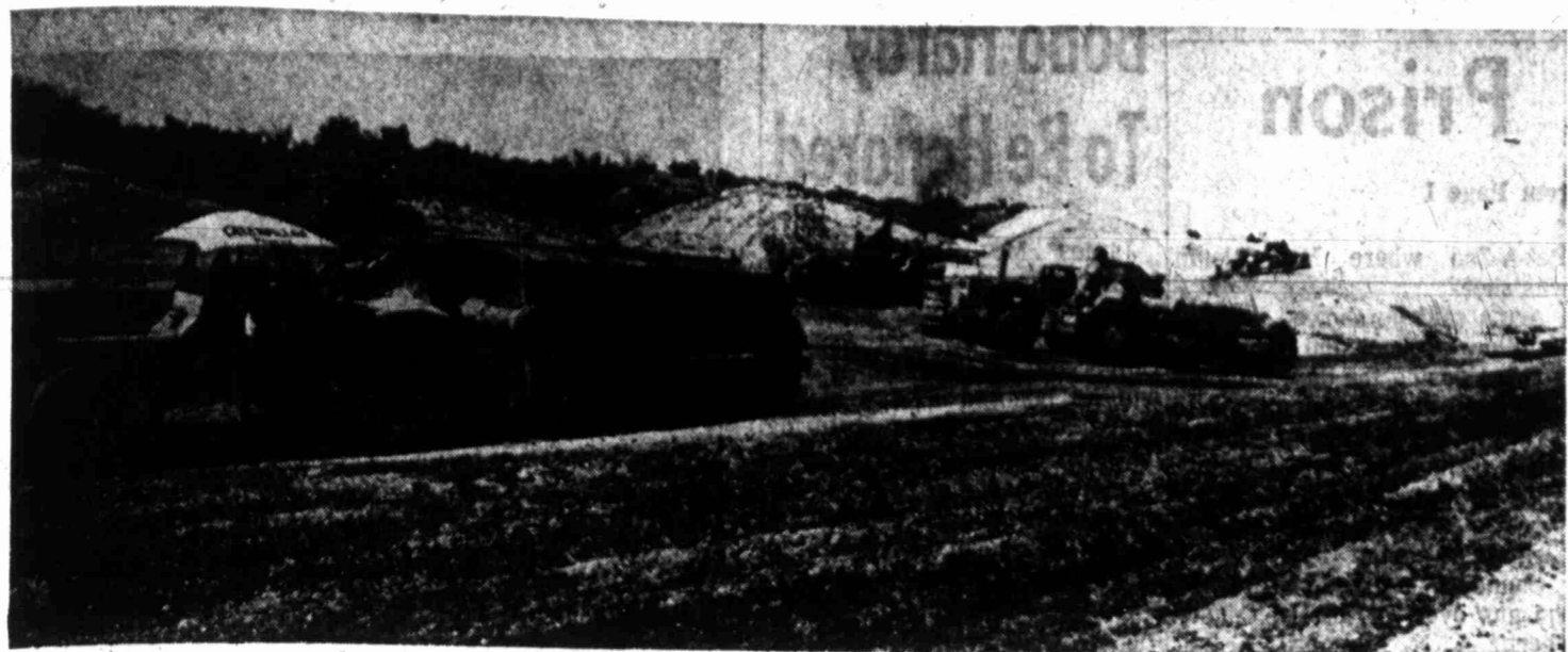
HIGHWAY CONSTRUCTION — Graders are at work on FM 700 where Strain Bros. workmen from San Angelo are busy widening the highway. The project is part of a highway improvement job contracted by the Texas Highway Department and should be completed in about a year. Work will also be done on culverts on US 87 South under the same project. (Photo by Lynn Kay Weaver)
