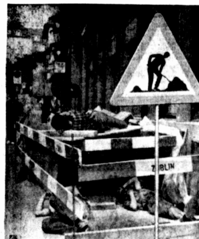
MEN AT WORK? — This scene at a street repair site in the Swiss city of Zurich resembles a sleep-in. Perhaps, the crew foreman went home for his siesta.
