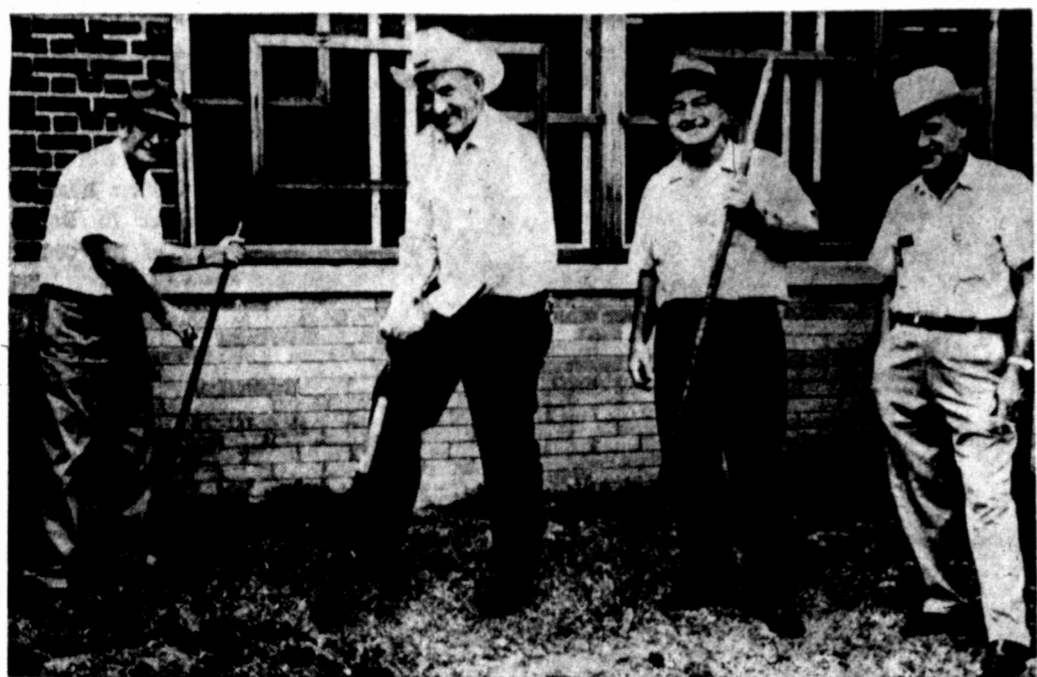
PORTABLE CLASSROOM—Increased enrollment at Kentwood Elementary put these four men to work this week moving in a portable classroom for a second sixth grade class. Amos Swindell, left, Nile Baily, Kelly Mize and Bill Gray are shown connecting gas lines between the classroom and the school building. The corner of the classroom is shown at Gray's right.
