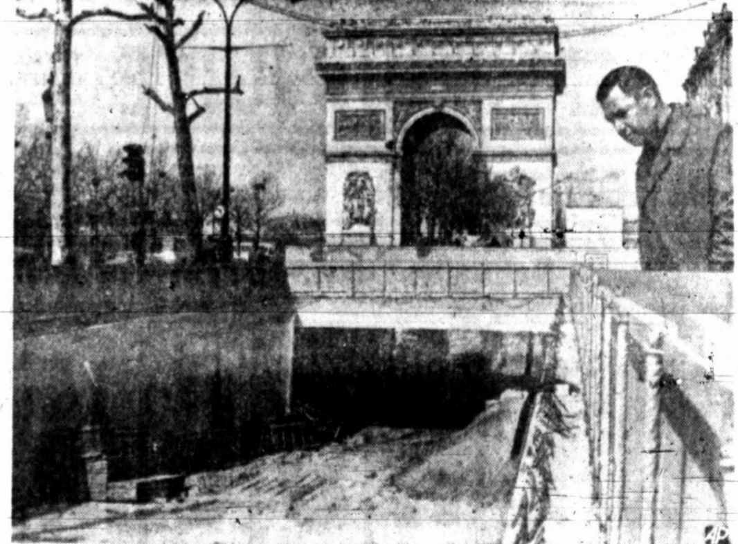
UNDER NOT AROUND — You're looking at the underpass that will permit vehicles to go under the Arc de Triomphe in Paris and relieve the auto congestion in the area.
