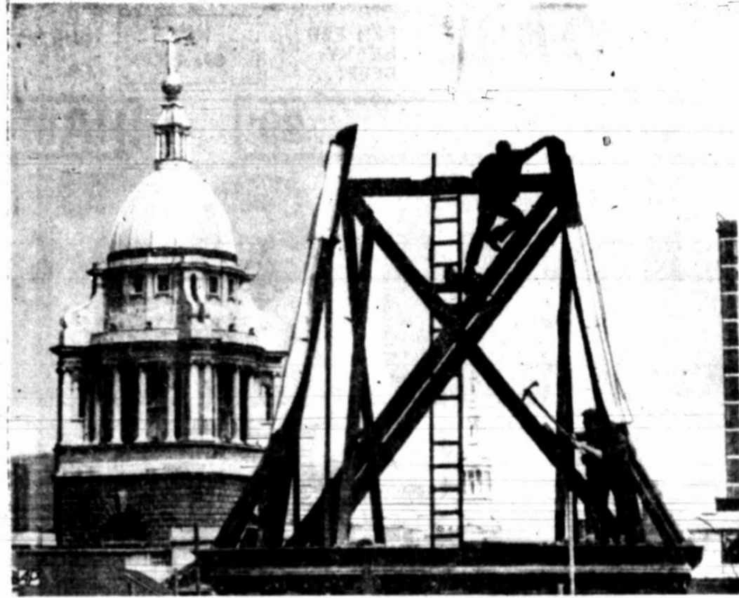
CHANGING SKYLINE — Workmen demolish last remnants of one of the towers on Memorial Hall in the City of London. Now visible as left is the dome of the Old Bailey. The Hall, to be replaced by an office block, was a conspicuous London landmark.
