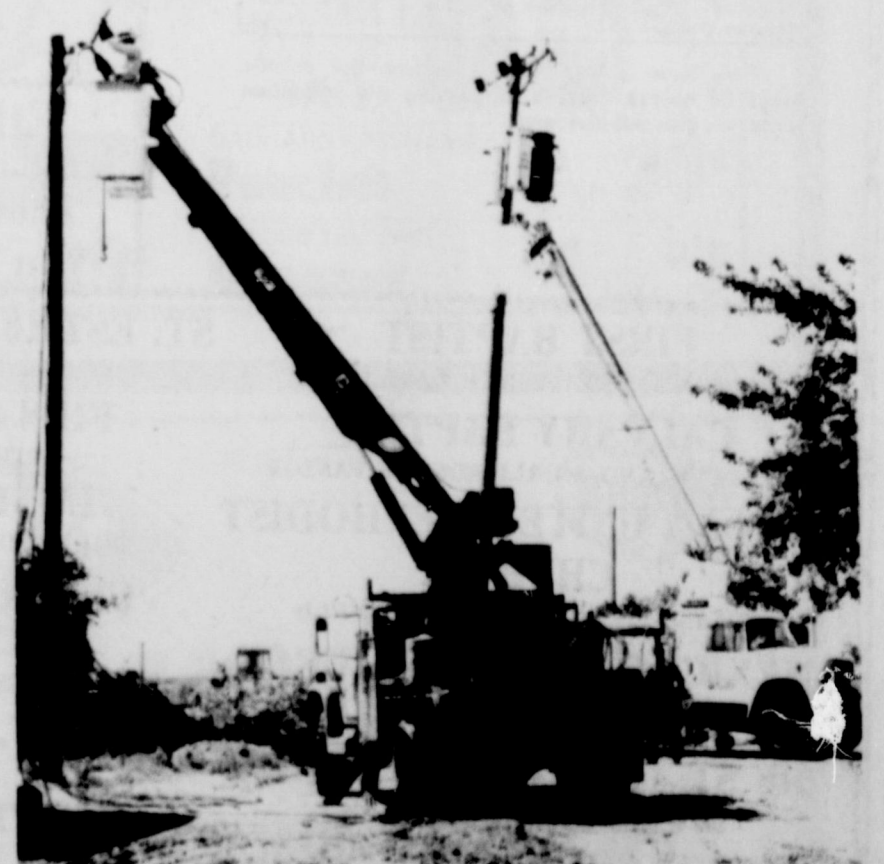
WIRING CHANGE....Southwestern Public Service Company employees are shown moving a pole and transformer on its system just off Fifth Street in Friona this past
