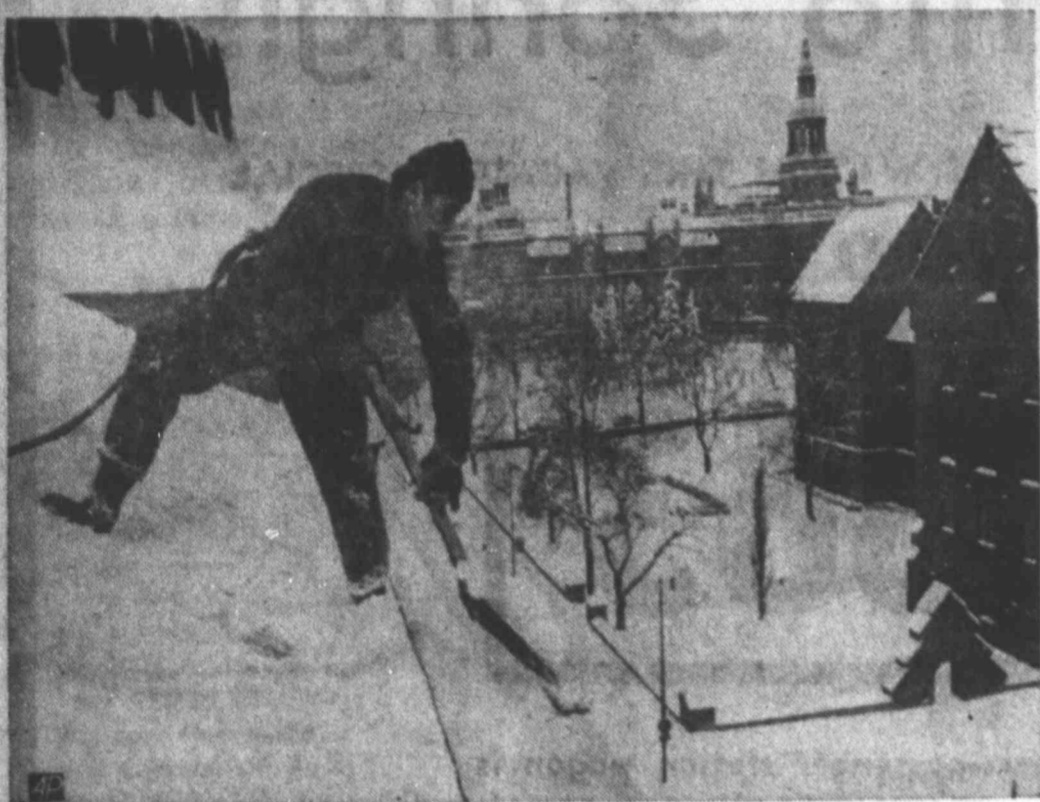
PRECARIOUS PERCH — A slip can be fatal for this worker who goes about his job of clearing snow from the slanted rooftops in Stockholm, Sweden. His only tie with safety is the rope around his middle secured to the rooftop. It's a long drop down.
