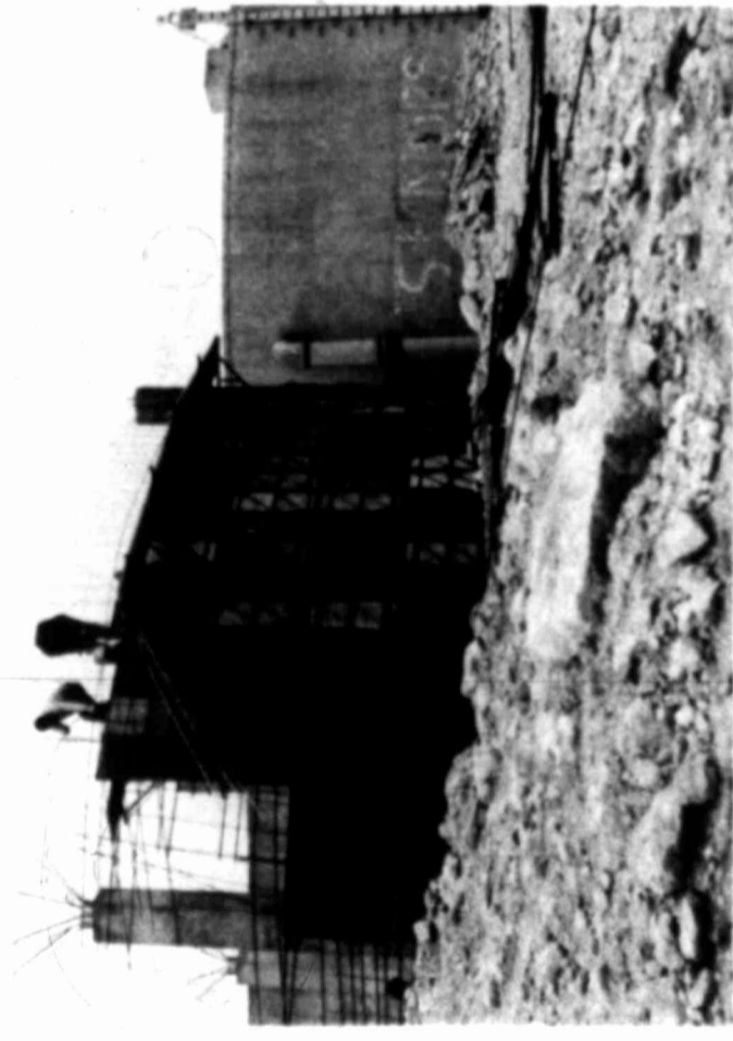
OUTSIDE . . . Construction moves ahead on this new water storage reservoir on top of a hill in the Edwards Heights area to insure that area an adequate water supply. It will hold 1,000,000 gallons when complete, and is also a part of our Master Plan program.
