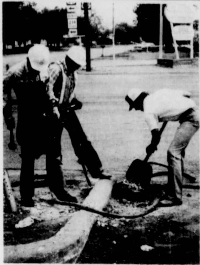
WORK BEGUN.... Highway Department employees began preparations this week to install a stop and go light at the intersection of Main Street and Highway 60. Installation is expected to be completed by early July, according to a spokesman for the highway department.
