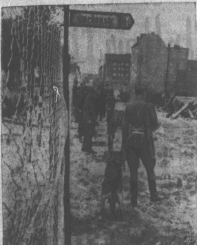
WALL WORK — East German soldiers, supervised by sergeant with police dog, set up part of the new border after apartment houses were removed in Berlin area.
