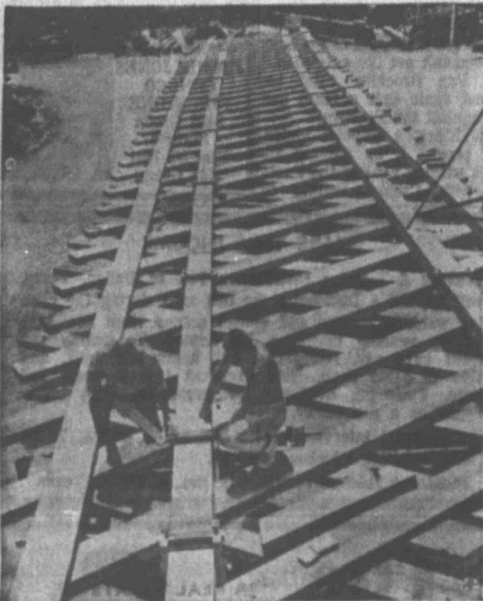
A DRY RUN — Workmen assemble a 150-foot span of a new covered bridge at Ashland, N.H. It'll be taken apart for trucking and location at Woodstock, Vt., site.
