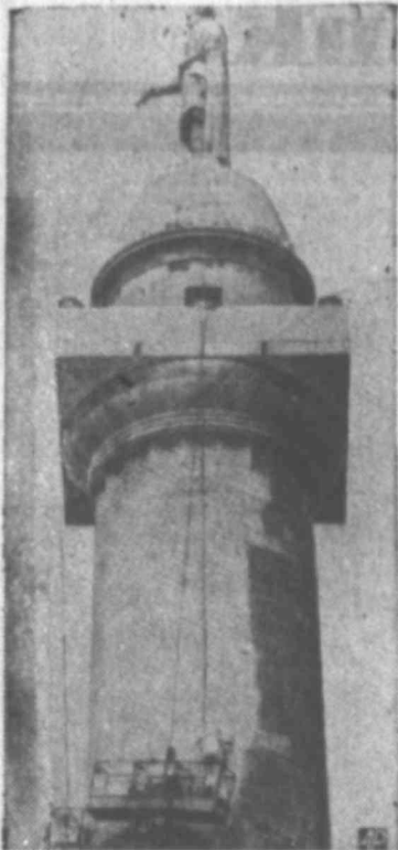
HIGH SWAB — Water under pressure is used to clean the Washington Monument in Baltimore. It was the first cleaning the 188-foot marble column received in 153 years.
