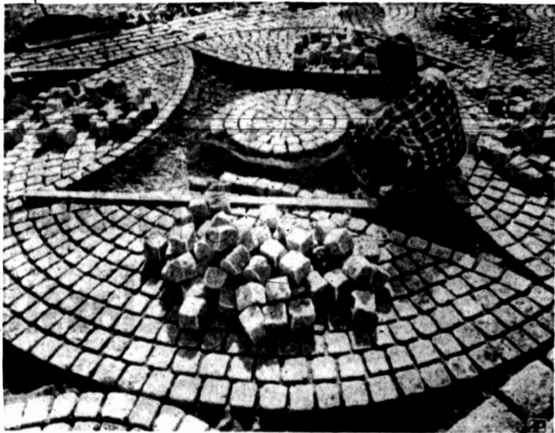
PATTERN IN STONE — Workman studies placement of granite blocks being laid by hand in intricate patterns for an unusual plaza at the State University of New York in Albany. The granite from South Carolina is cut and shaped by the hammer and chisel.
