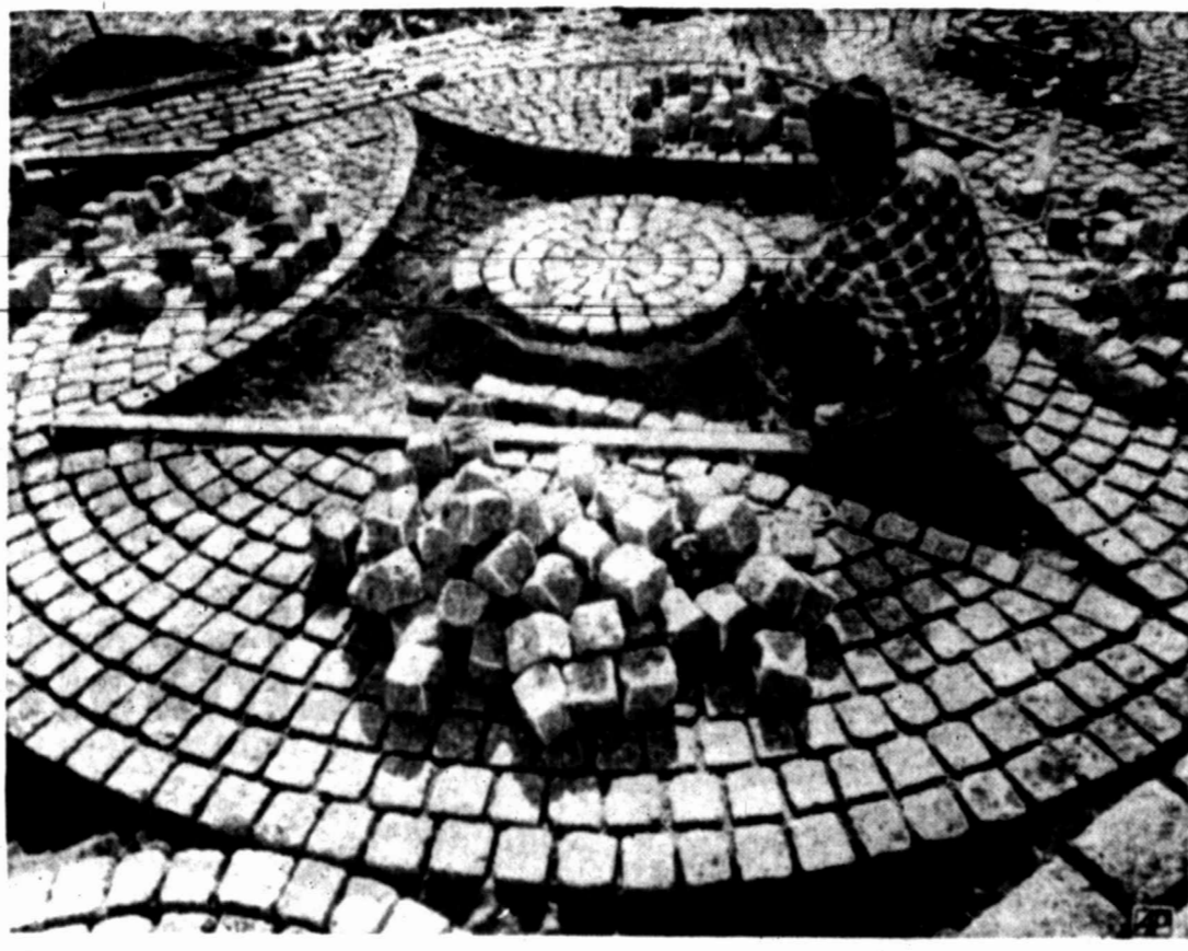
PATTERN IN STONE — Workman studies placement of granite blocks being laid by hand in intricate patterns for an unusual plaza at the State University of New York in Albany. The granite from South Carolina is cut and shaped by the hammer and chisel.
