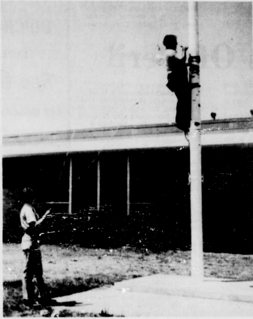
UP A POLE... A workman is shown applying a fresh coat of paint to the flagpole at Friona High School. The job was accomplished on Thursday despite high winds.
