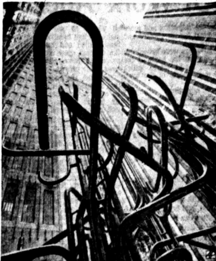
DIFFERENT TWIST — Unusual array of 400 individual sections of stainless steel pipes with 42 symbolic burners fronts 25-story home of the Atlanta Gas Co.
