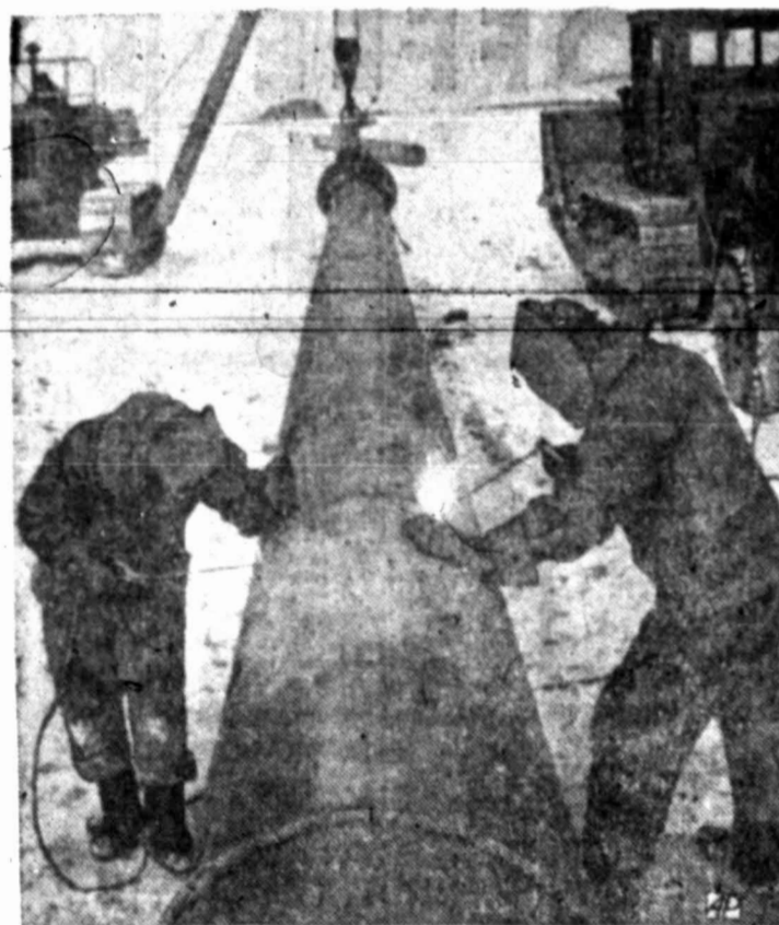
ANOTHER LINK — Welders work on section of pipeline which will bring gas to Alma Ata in Southern Russia.
