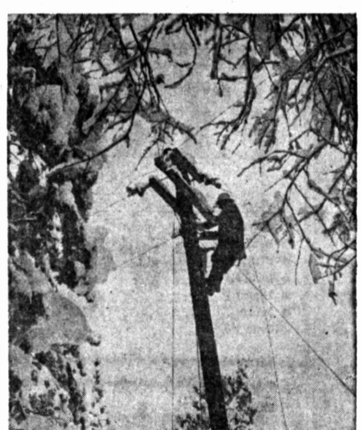
UP AND AT 'EM — Despite the rough weather, a lineman repairs a distribution line taken out by a falling pine in Grass Valley-Nevada City, Calif. area.
