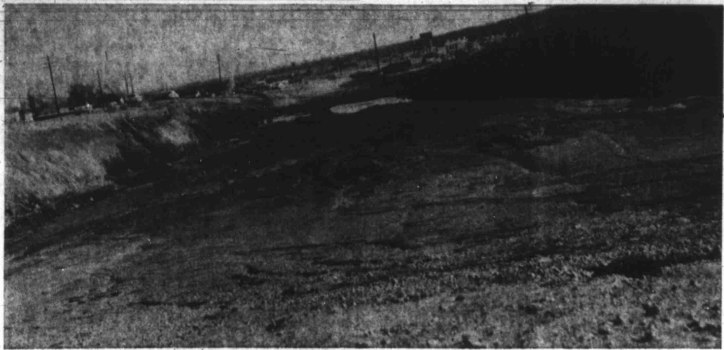
FM 700 BEING TRANSFORMED INTO FOUR-LANE HIGHWAY Channel for underpass at intersection with US 87 being excavated (Photo by Sam Blackburn)
