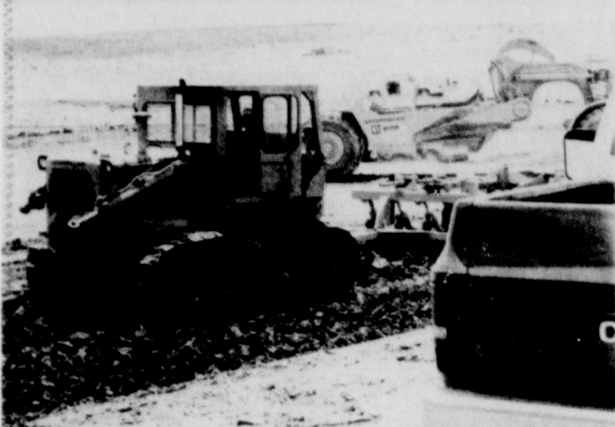
BUILDING A DAM... Heavy machinery at the Lazbuddie dam site has been active since June to construct a dam on the Running Water Draw near Lazbuddie. The dam is being built for flood control and will cost an estimated $1.33 million. It will take 1½ years to complete the project. (Star Photo)
