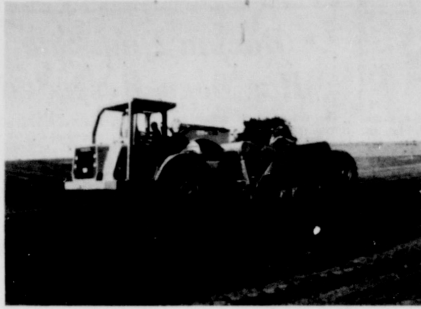
WORK BEGUN....Mammoth earth-moving equipment began working on dam site number three on Running Water Draw near Lazbuddie this week. The carryall was in the process of removing the topsoil at the dam site.
