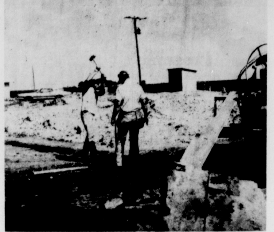
CONSTRUCTION BEGUN...Builders have started work at the Lazbuddie School on what will be a new gymnasium, concession stand,
