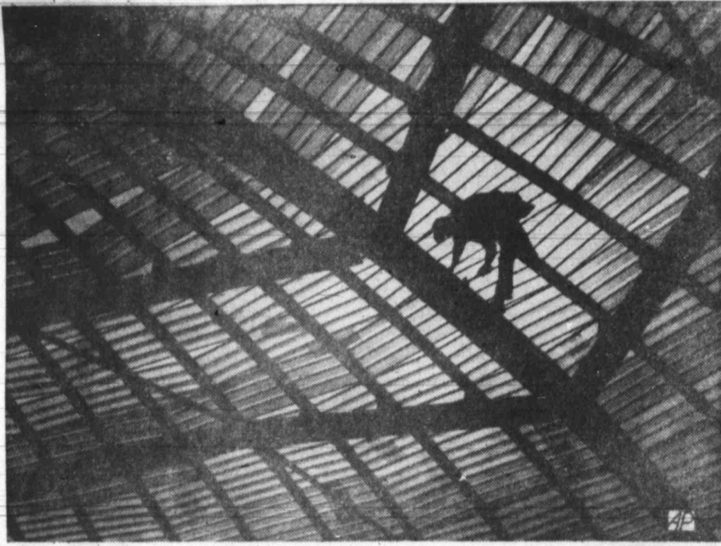
RISE IN THE WEST —Workman is silhouetted on roof of the Rondelle theater at Racine, Wis. The edifice, which was part of the New York World's Fair, is being reassembled on grounds of the Johnson Wax company as a Midwest tourist attraction.
