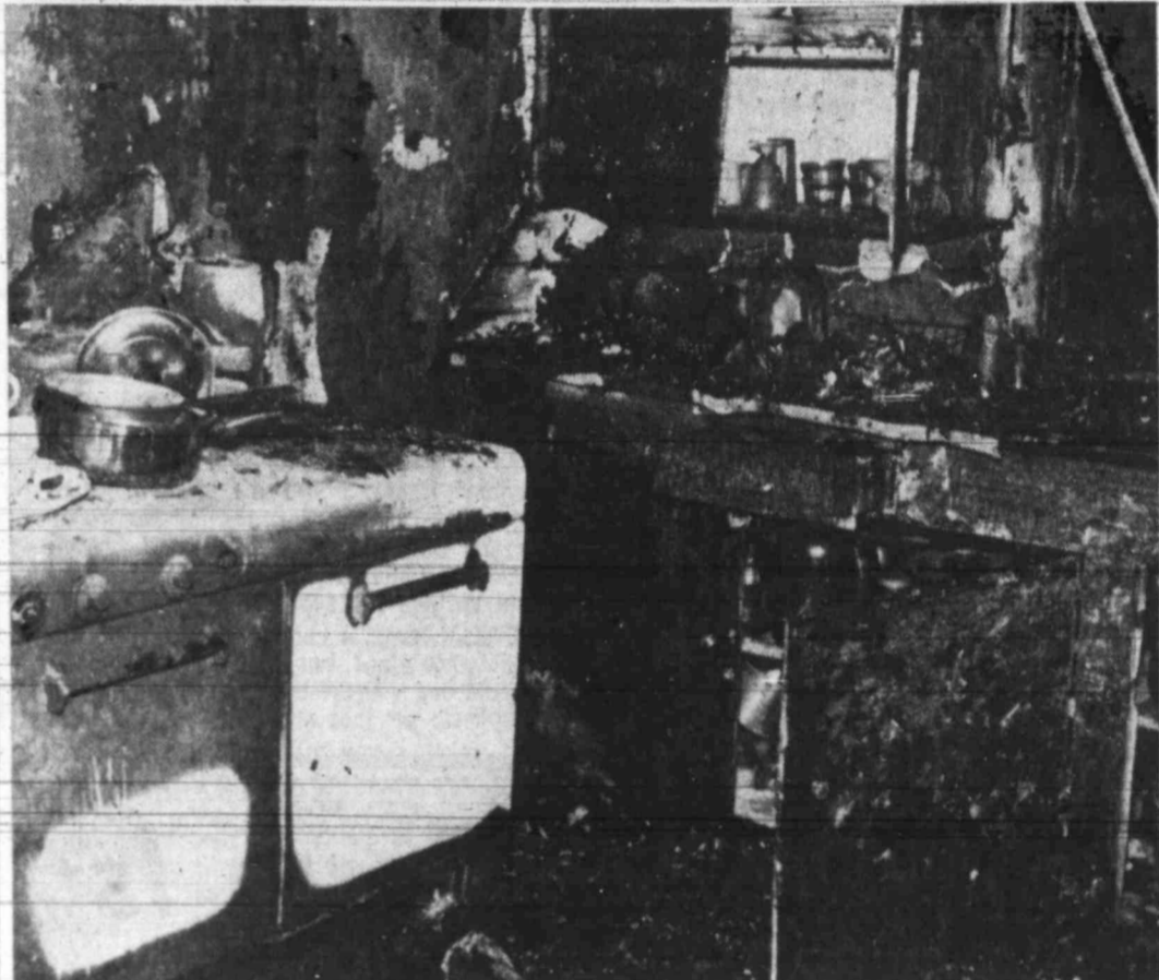
Fire Sweeps Through House
