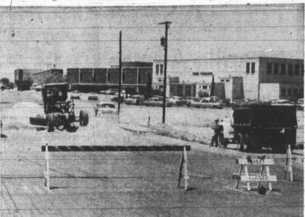
Improving Drainage. Eleventh Place, in the high school area, at Young Street, has been blocked since Monday as City of Big Spring crews have been lowering the street level, to match the drainage provided by a storm sewer installed by the school district. Ernest Lillard, public works director, said the work should be completed by late Thursday. The city is doing the dirt work and the school district will pay for the paving, which will be done by a contractor. The street will be temporarily closed till Friday when the topping is put on the street. (Photo by Frank Brandon)
