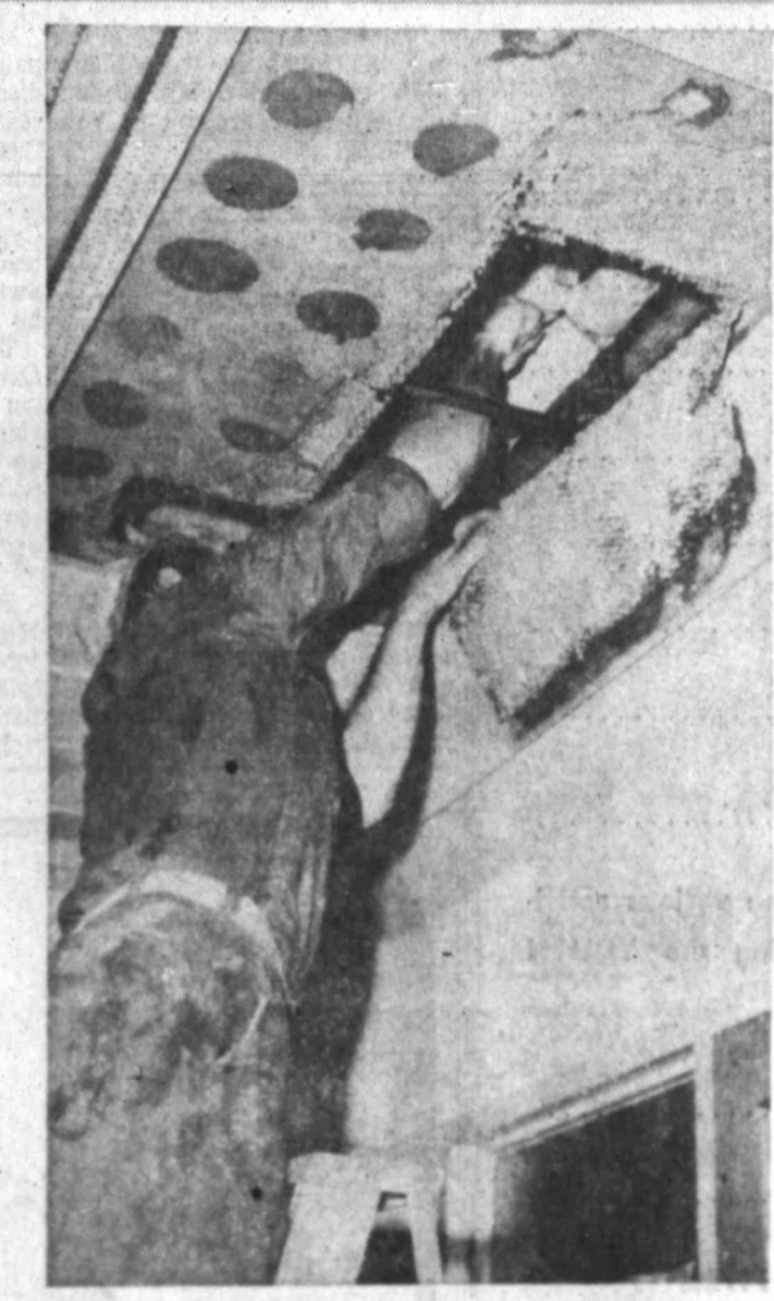
IT RAINED IN THE COURTHOUSE TODAY Burst water line in third floor ceiling creates minor flood
