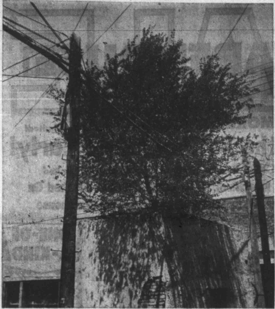
(Photo by Sam Blackburn) ROOFTOP'S NO PLACE FOR AN ELM TREE TO GROW! Nevertheless, that's where this towering tree has sprouted
