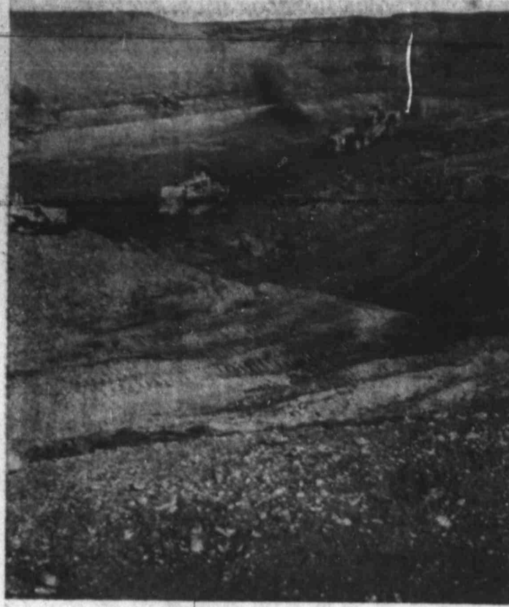
CRADLE FOR A HUGE BOWL Elbow of service spillway to rest here
