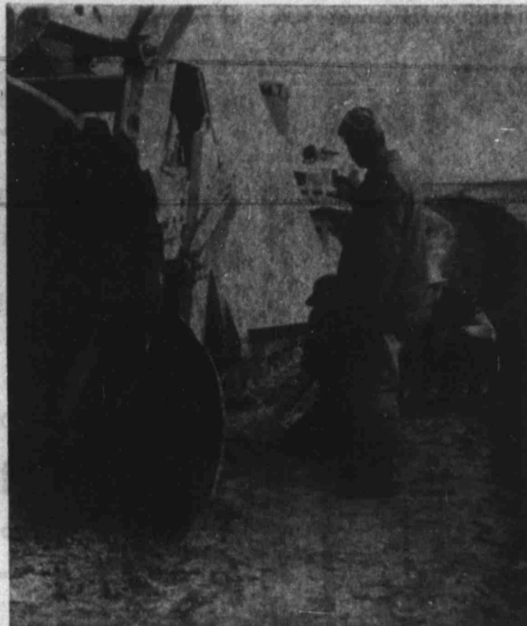
LOADER READY TO GOBBLE UP EARTH Discs toss cubic yard per minute on conveyor
