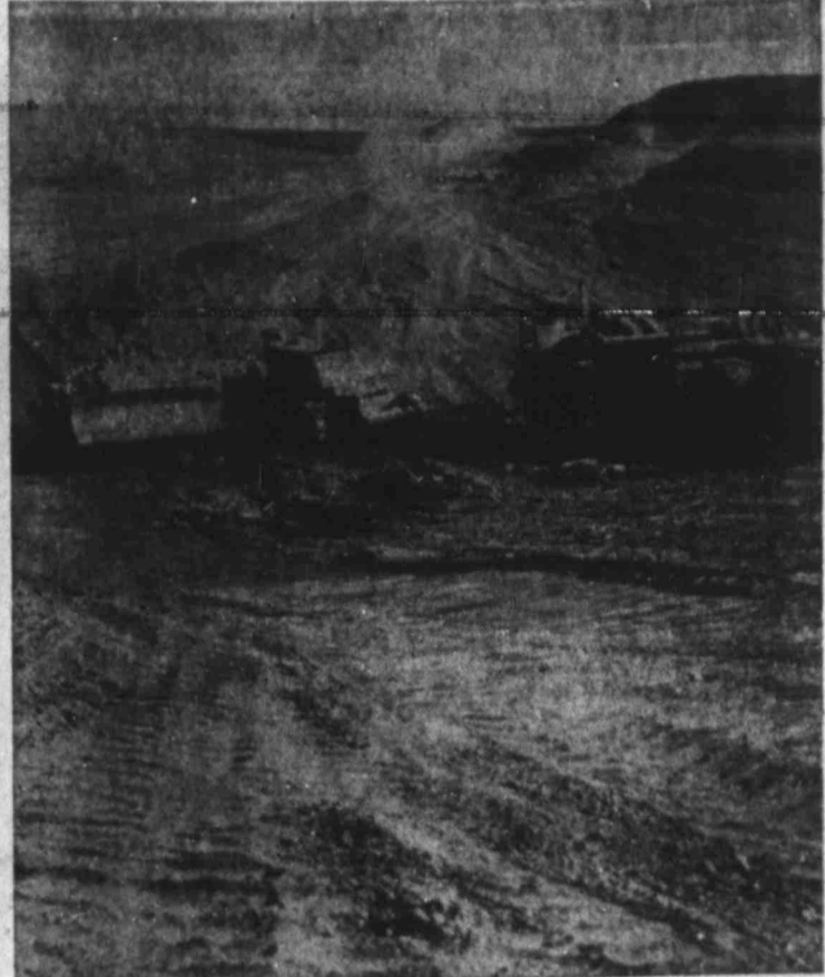
DIG AND BACK-FILL FOR CORE OF DAM Excavation filled with clay, wetted-rolled
