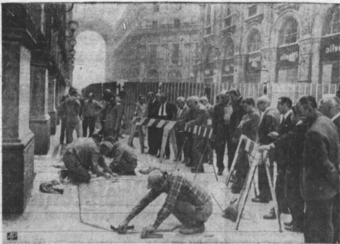
SETTING THE STONES — There are plenty of "sidewalk superintendents" as workers restore mosaic flooring of famed Milan Gallery. Structure is almost 100 years old.
