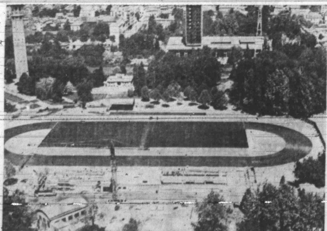
SETUP FOR SPEED — Panoramic view shows the ice rink under construction at Grenoble, France, where speed skating competition will take place in 1968 Winter Olympics.
