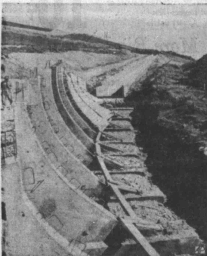
A HIGH RUN — The concrete settings for the bobsled track on the Alpe d'Huez above Grenoble in southern France are readied for the 1968 Winter Olympic Games.
