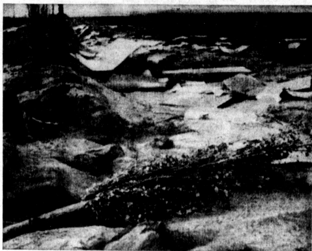
Broken Irrigation Ditch
