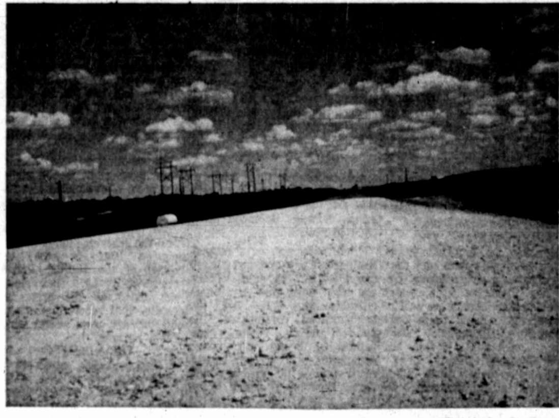
FM 700 NORTH PUSHES TOWARD COMPLETION New highway link slated to be finished in early October
