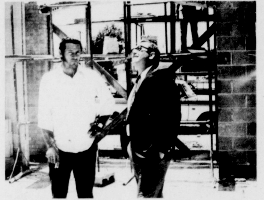
TAKING SHAPE.... Contractor Sony Blair and assistant postmaster Dewayne Howard watch as workmen begin installing the roof on Friona's new post office building. In
