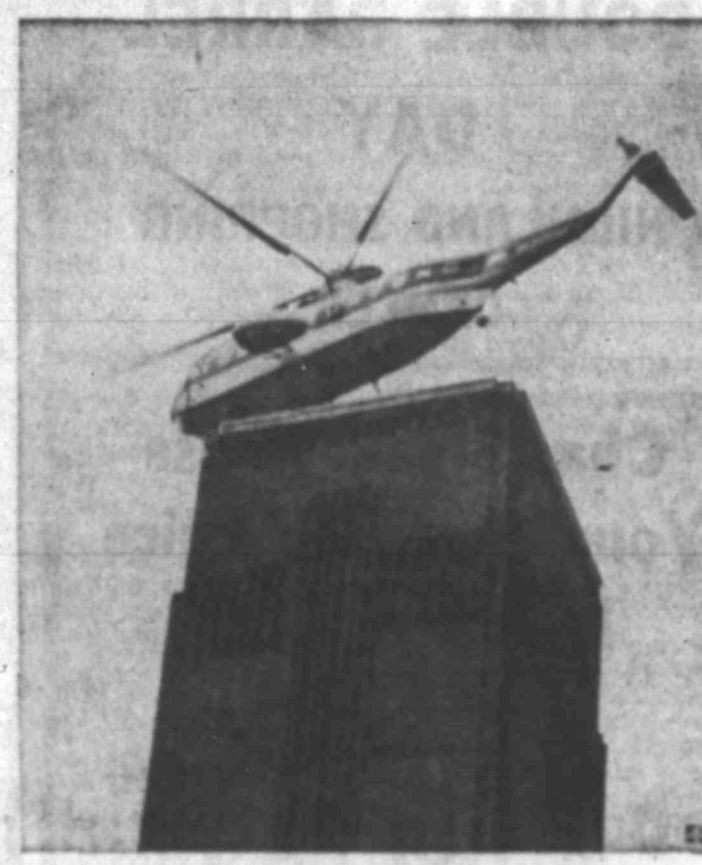
A HIGH LIFT —Helicopter, acting as a crane, waits above 300-foot high Bankside Power Station in London to effect transfer of half-ton chimney cylinders.
