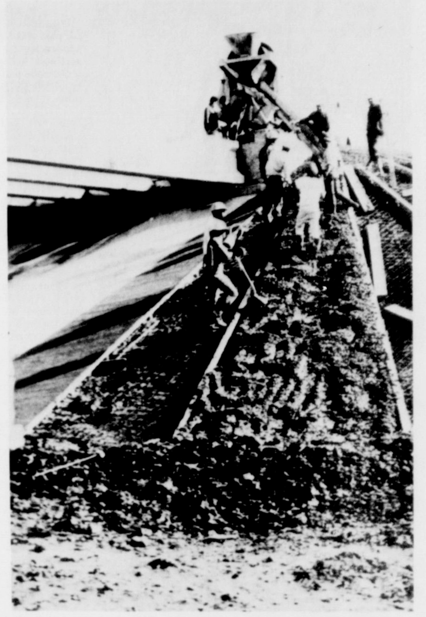
BRIDGE WORK....Construction continues full pace on the overpass which is spanning Santa Fe Railway south of Friona on Highway 214. Pre-stressed concrete beams were laid to span the bridge this week. Workmen are shown pouring concrete on the approach to the bridge. Officials say the bridge could be open in six months.
