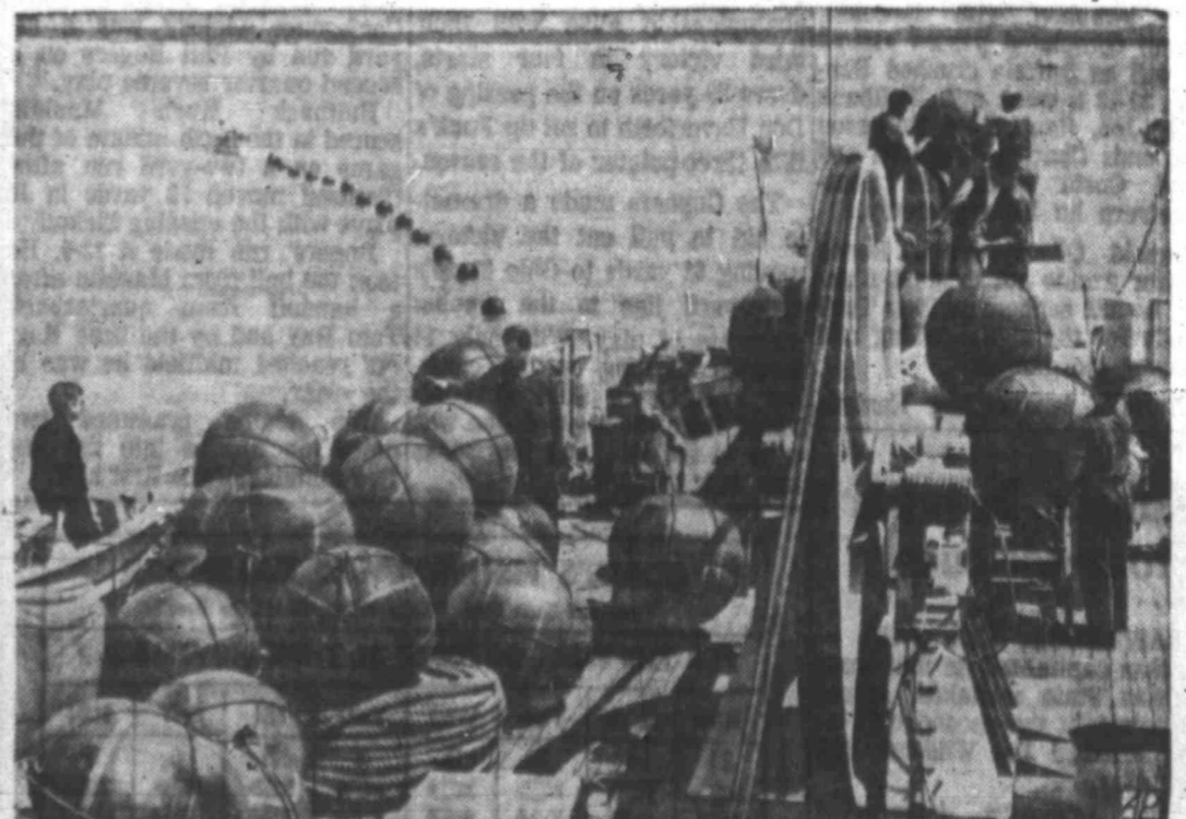
AID FOR THE LINE — Heavy-duty balloons are utilized by a French cable-laying vessel in shallow water off the Brittany coast. The big balls were used to hold cable in place during laying operations. Communications line links the U.S. with France.
