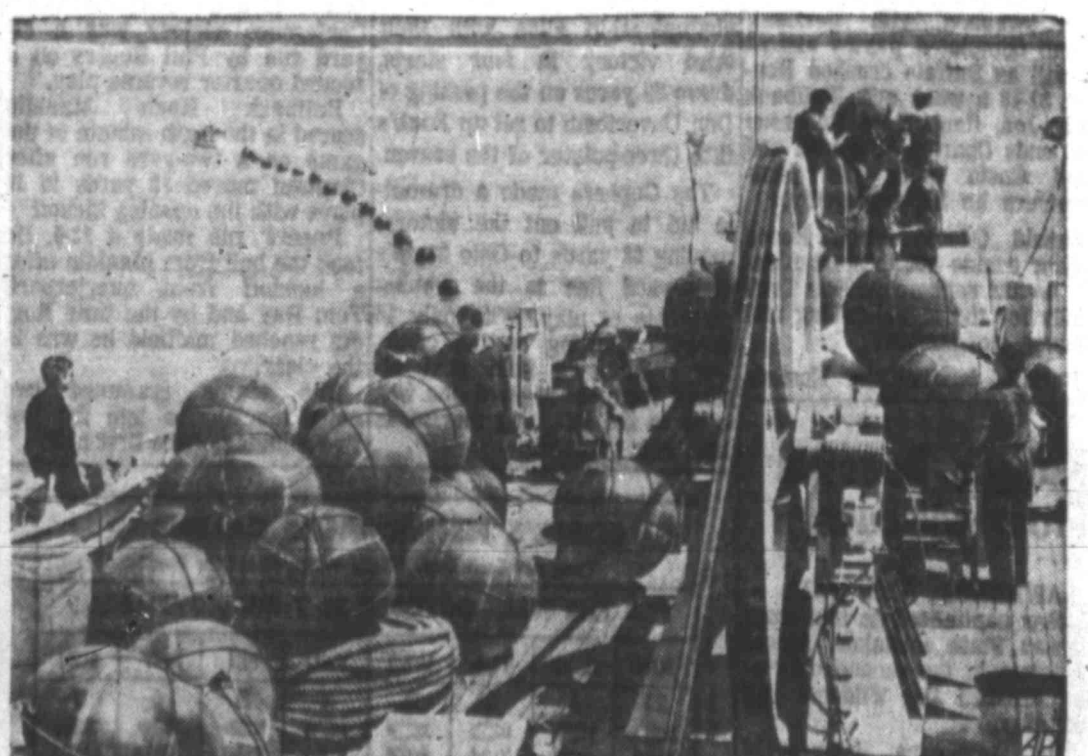
AID FOR THE LINE —Heavy-duty balloons are utilized by a French cable-laying vessel in shallow water off the Brittany coast. The big balls were used to hold cable in place during laying operations. Communications line links the U.S. with France.
