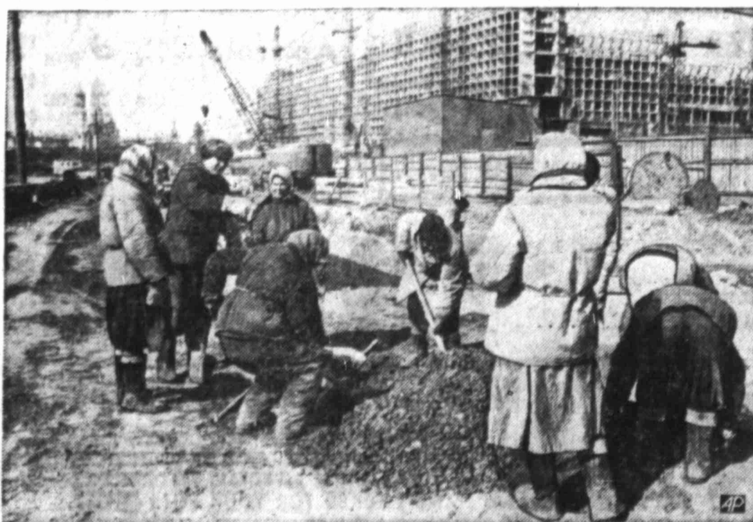
SHARING THE LOAD — Equality of sexes means something in Russia where even heavy manual jobs are open to women as well as men. Here, a group of heavily padded female laborers mix concrete on the site of the new Rossiya Hotel, background, in Moscow.
